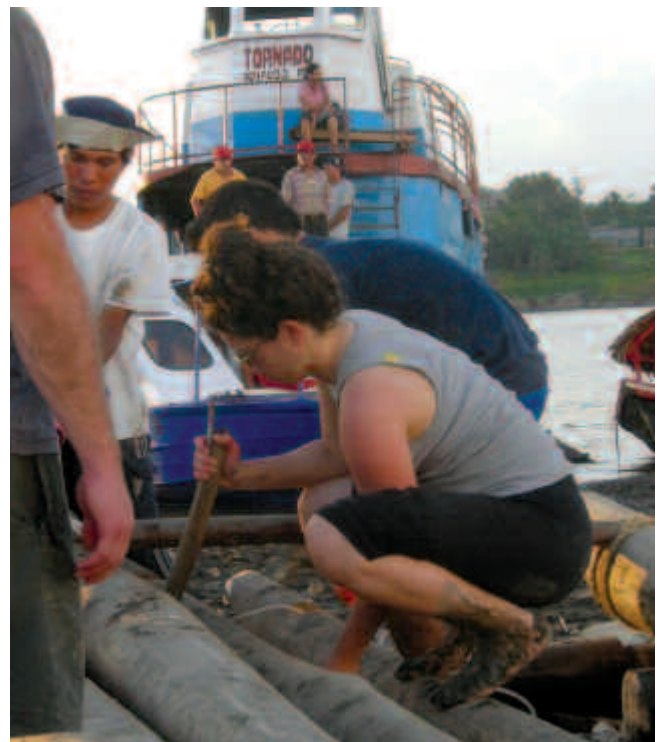
Leora building the raft she used to compete in the 112-mile Amazon Raft Race.
